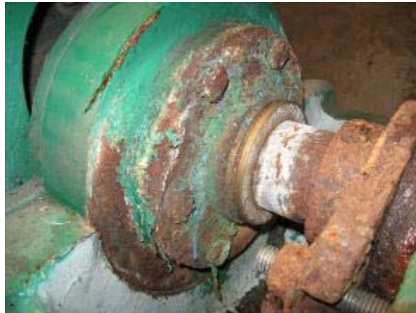
Photo 3.18 – Circulating Water Pump 6-2
