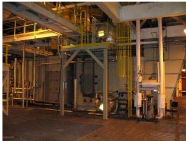
Photo 3.6 – Heat Recovery Steam Generator
