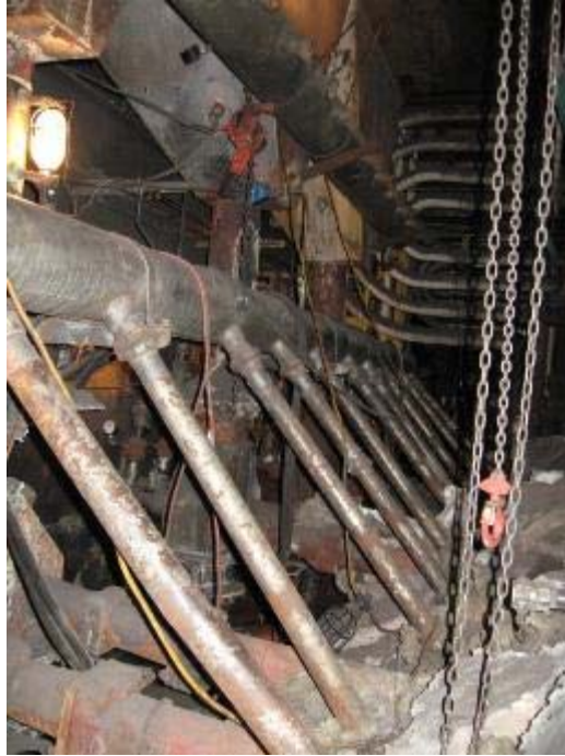
Photo 3.3 – Ash Rejection Nozzles
