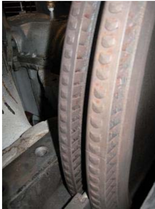
Photo 3.12 – Pump 6 Steam Turbine
