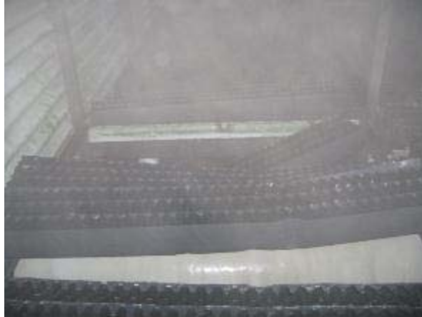
Photo 3.24 – Cooling Tower Drift Eliminators
