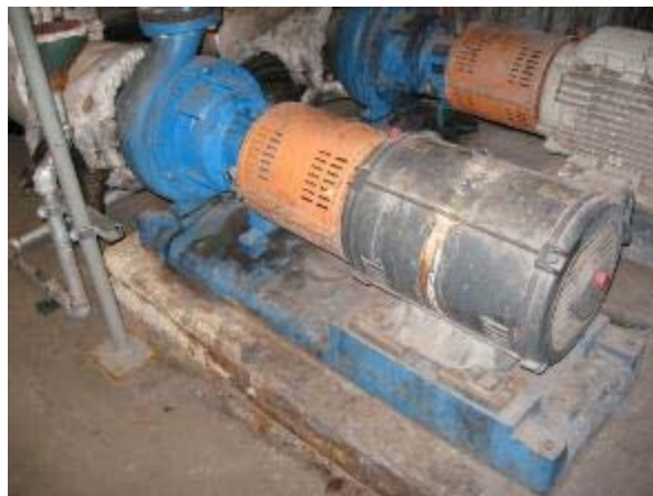
Photo 3.14 – Condensate Forwarding Pumps 1 & 2
