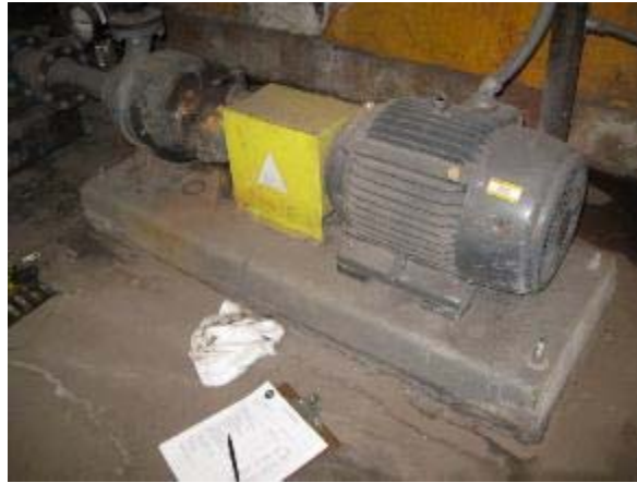
Photo 3.13 – Condensate Elevation Pump 3
