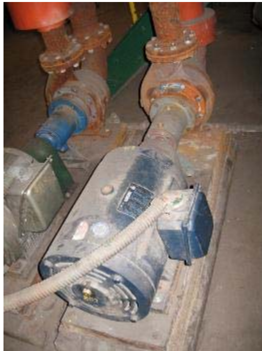
Photo 3.17 – Raw Water Pumps 1 and 2
