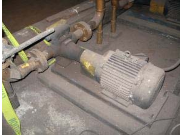
Photo 3.19 – Fuel Oil Pump 4
