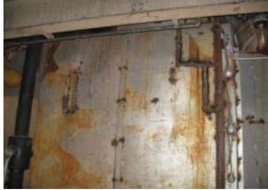
Photo 3.1 – Boiler 3 Casing “Patches”
