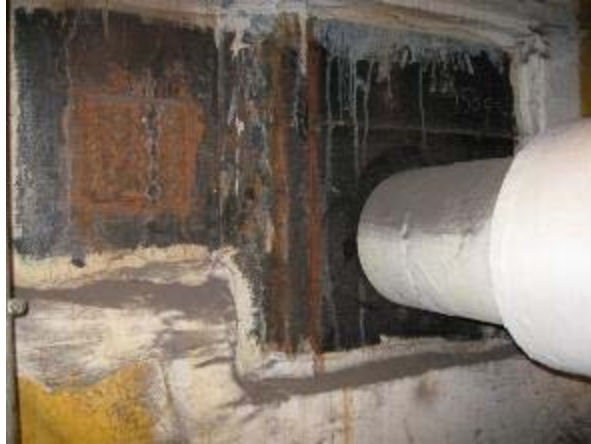
Photo 3.21 – Condensate Return Tank 1
