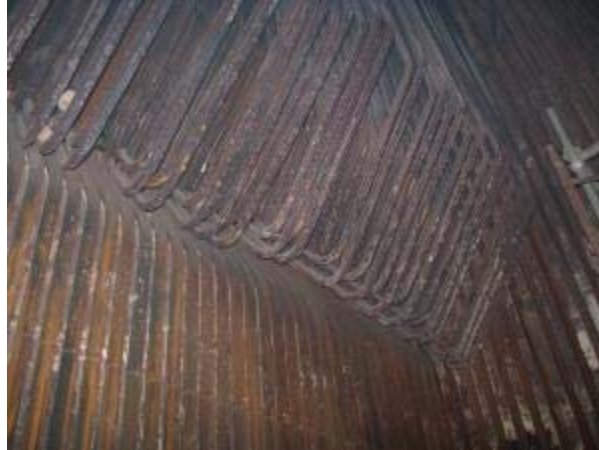
Photo 3.9 – Boiler 5 Superheater Tubes
