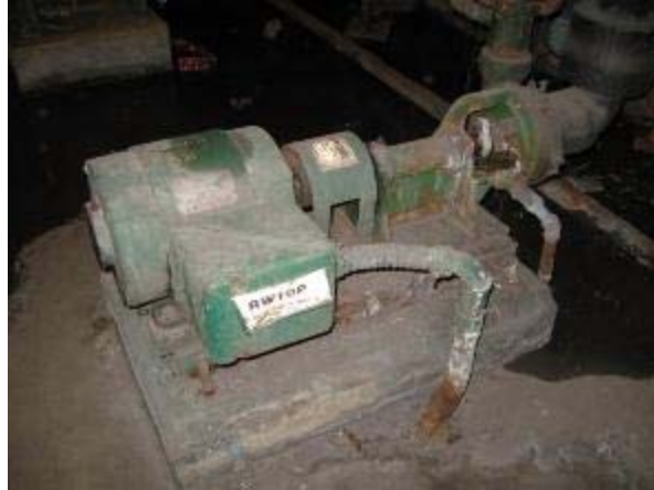
Photo 3.16 – City Water Booster Pump 1
