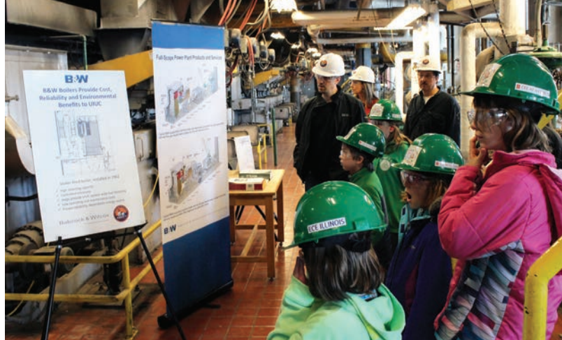
Guided plant tours and poster displays gave visitors an insider's perspective on the production of heat and power at Abbott Power Plant.
